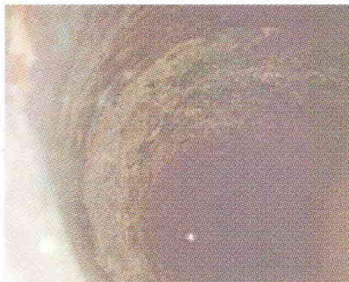
Pic 5 Looking down a Roman well situated on the Northern edge of the Parish
